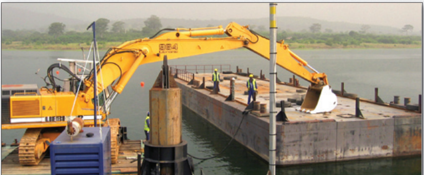
Barges and backhoe being readied for a timber salvage operation in the Afram Arm of the Volta Lake.
